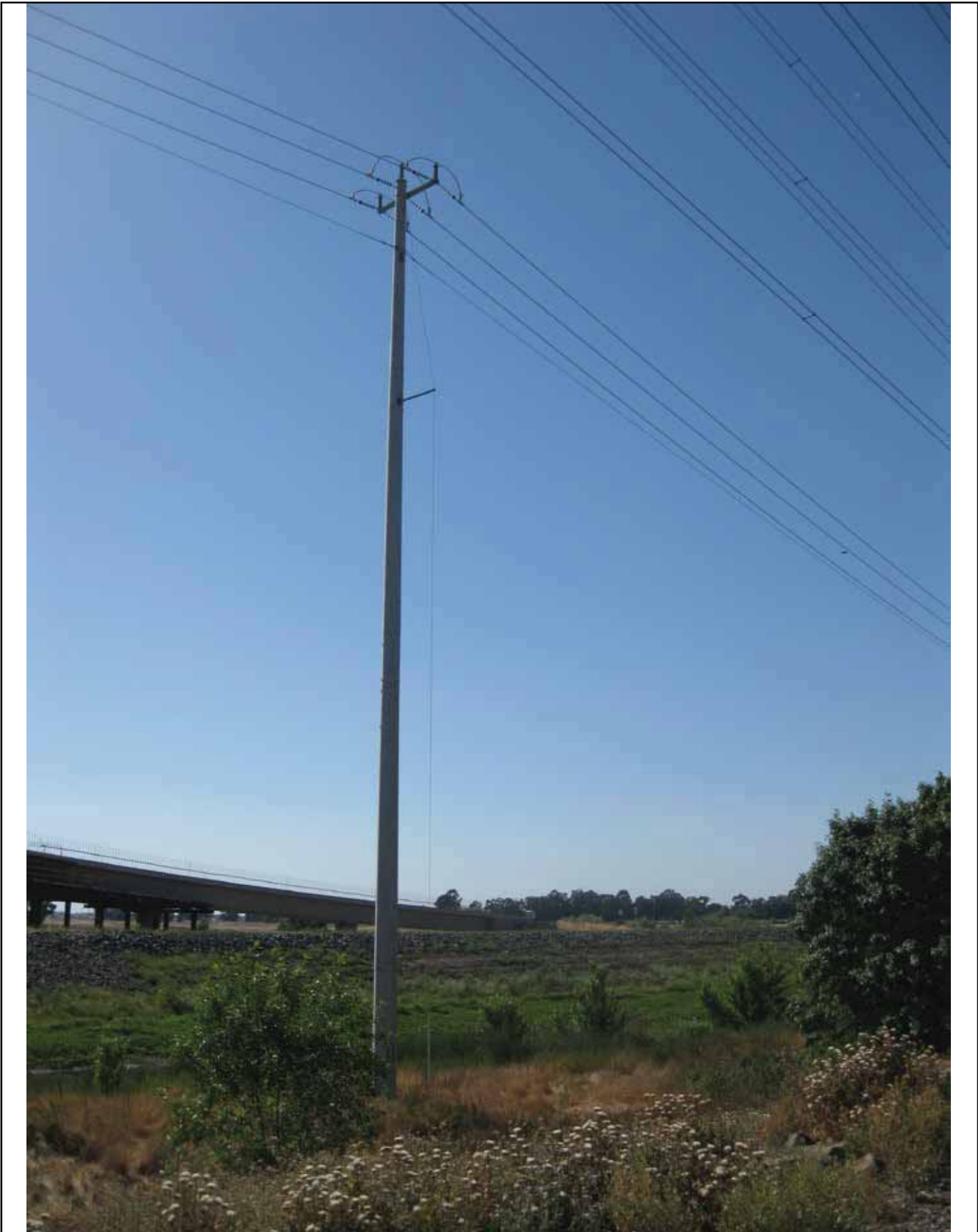
EXHIBIT 11: Typical 69 kV Tubular Steel Pole (TSP) to be installed as part of the proposed project
